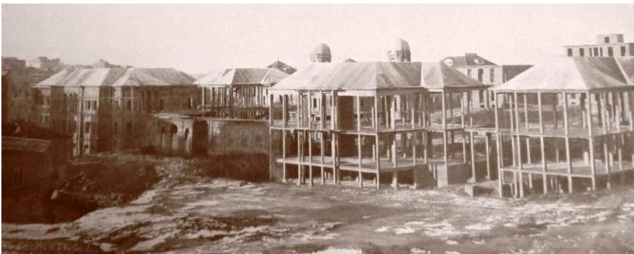
Figure: the building site of San Martino hospital in Genoa, where reinforced concrete frames are infilled with thick masonry stone walls.
